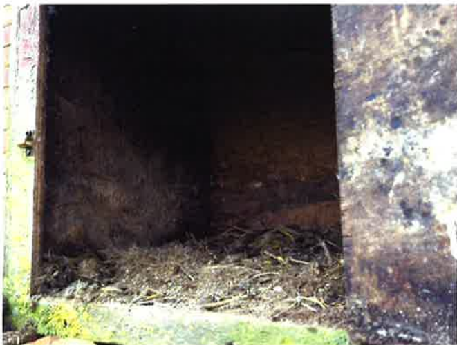
Heckington Pumping Station (3): Before
