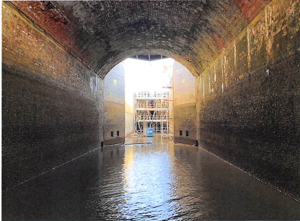
Photographs looking through the drained down Black Sluice Navigation Lock (Boston) and works on the navigation sea doors (October 2020).
