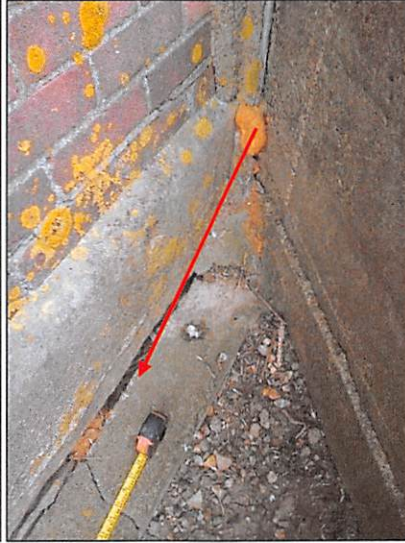
Photograph 2 Cracking between the pumping station building and the retaining/wing wall. Expanding foam used as a temporary measure to infill the crack
