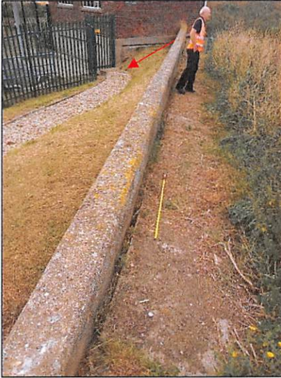
Photograph 1 - Cracking parallel to the concrete retaining/wing wall. Indicating settlement of the soils to the south (right of photo) of the wall. Taken from the west side of the pumping station, looking east
