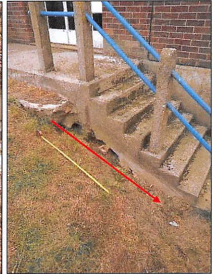
Photograph 6 Settlement of the soils beneath the stairway leading into the pumping station building. Photograph taken from the eastern side of the building looking westwards
