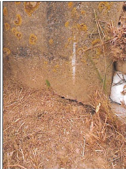
Photograph 5 Settlement of soils beneath the pumping station building foundation
