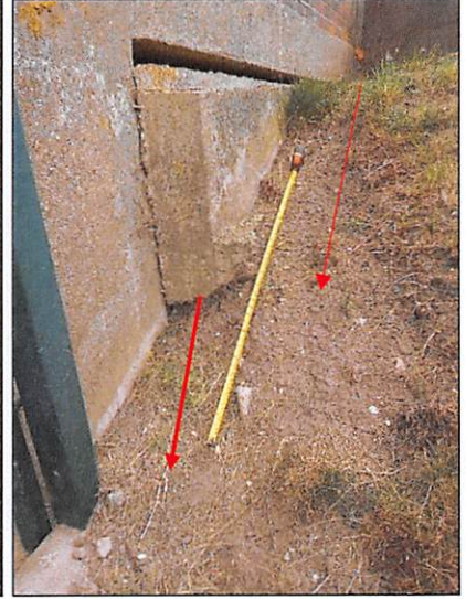
Photograph 3 Exposed and displaced foundation slab beneath the pumping station building, indicating settlement of the underlying soils
