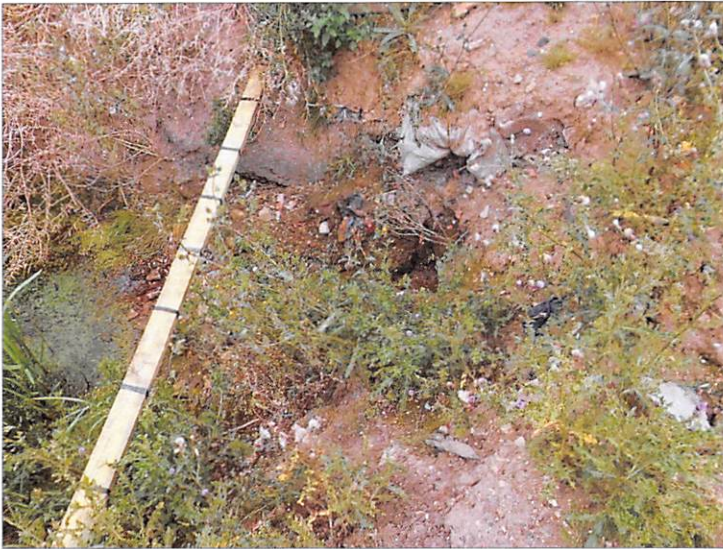
Exposed underground electric cable (secured by Western Power Nov 2020)
