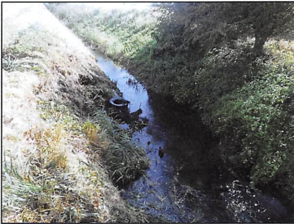
Previous control structure collapsed September 2020
