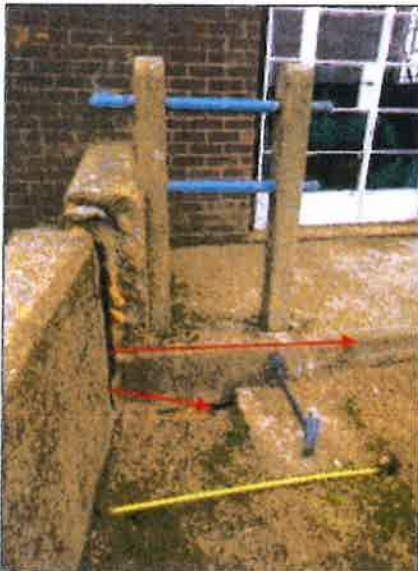
Photograph 4 - Displaced flood wall and settlement beneath concrete slab
