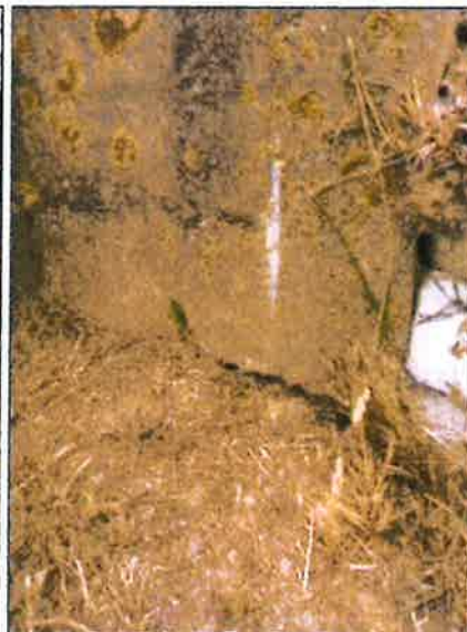
Photograph 5 - Settlement of soils beneath NE corner of pumping station building
