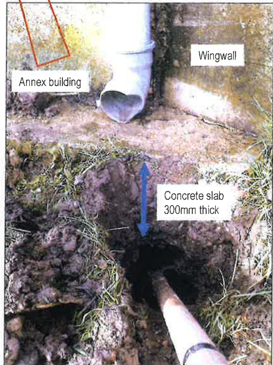
Hand Pit HP03 excavated on the southern (highwater) side of the pumping station/annex building. Hand pit terminated upon encountering pile foundation beneath capping beam/slab.
