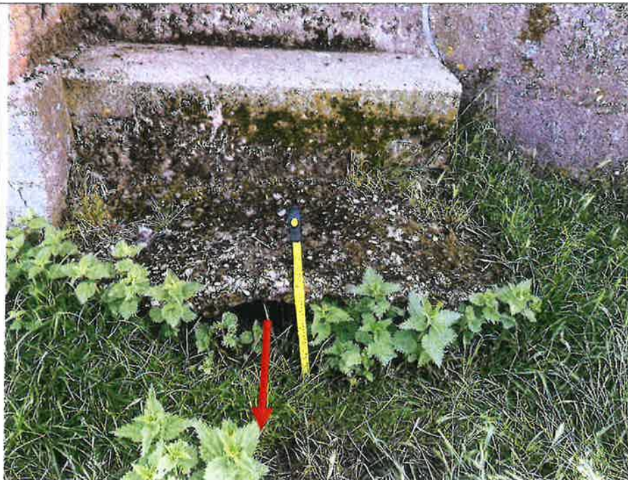
Photograph 2 - A void present beneath the bottom of the concrete steps to the west side of the pumping station as a result of ground settlement. Water has been noted to flow through this void during high water levels. Arrow denotes seepage water flow.
