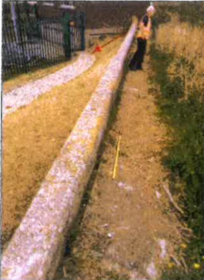
Photograph 1 - Cracking parallel to the flood wall. Indicating settlement of the soils southward (right of photo) of the wall.
