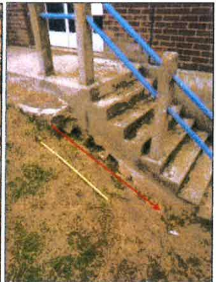
Photograph 6 - Settlement of the soils beneath the stairway leading into the pumping station building.
