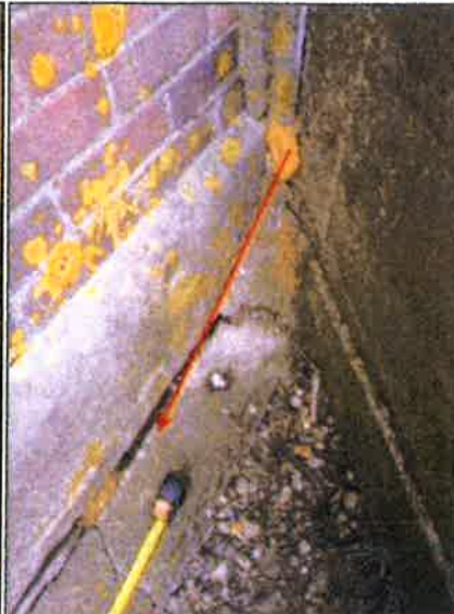
Photograph 2 - Cracking between the pumping station building and the flood wall. Expanding foam used as a temporary measure to infill the crack.
