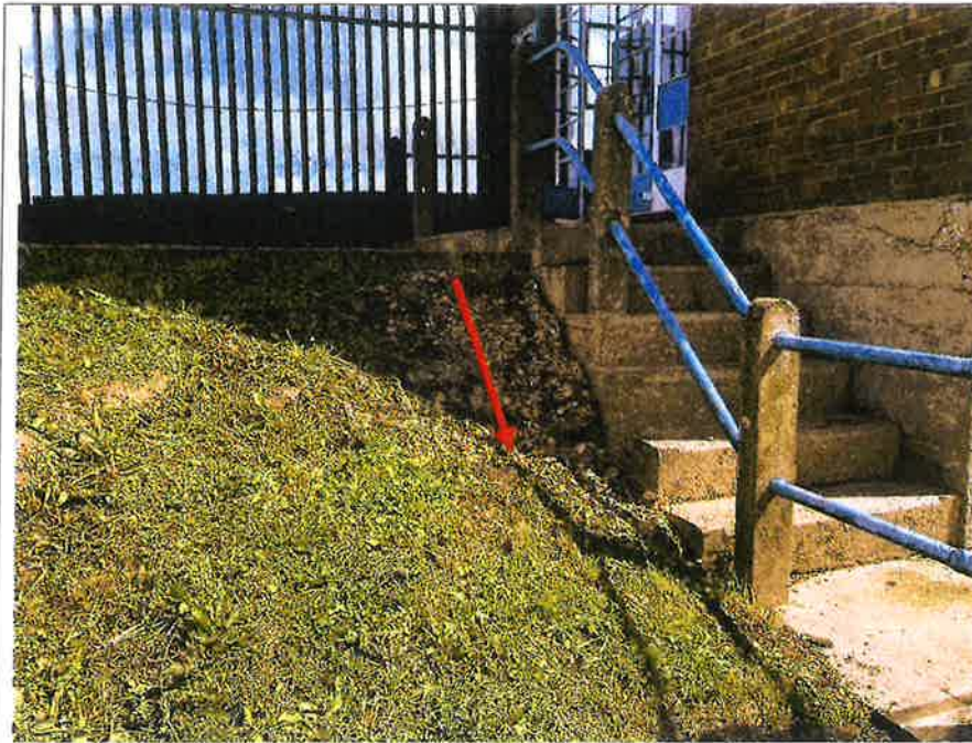
Photograph 1 - West side of pumping station. Settlement of the soils beneath the stairs leading into the pumping station building. Photograph taken looking north. Arrow denotes seepage water flow.
