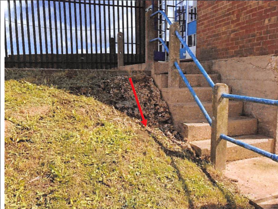
Photograph 1 - West side of pumping station. Settlement of the soils beneath the stairs leading into the pumping station building. Photograph taken looking north. Arrow denotes seepage water flow.
