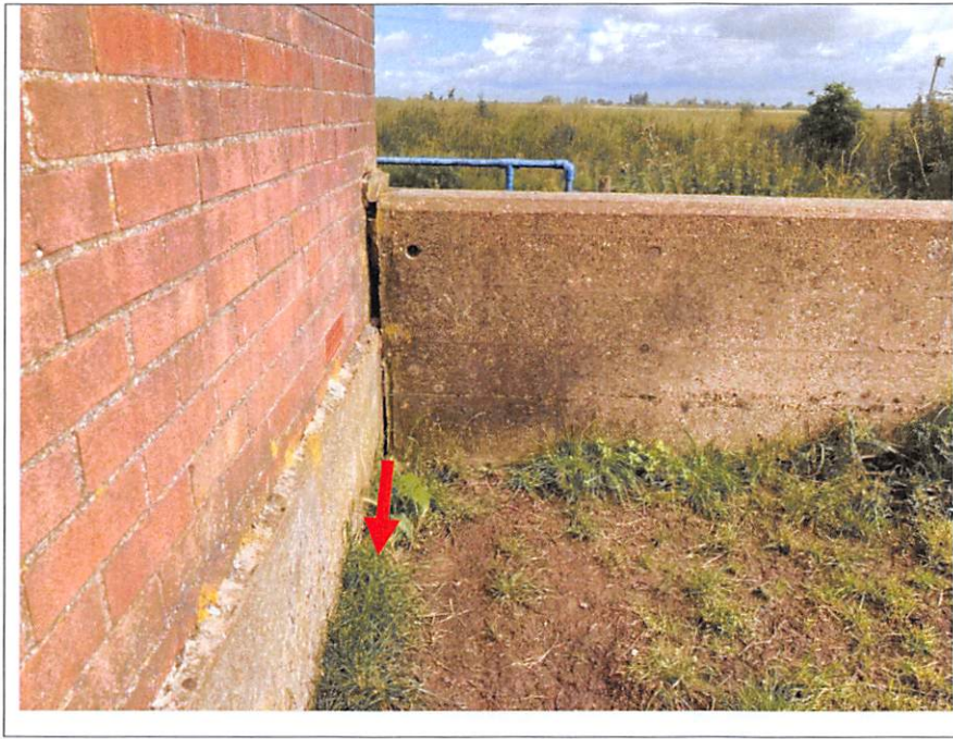
Photograph 5 - Eastern side of pumping station looking north. Wingwall has moved downwards and away from the building to leave a gap through which water flowed. Arrow denotes seepage water flow.
