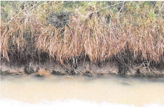
Silt exposed at north bank toe.
