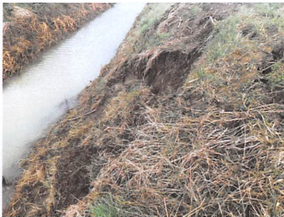
Bank slip near sett
