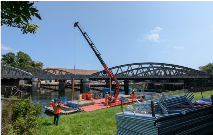
A barge equipped with a crane that will be used during the Grand Sluice refurbishment preparatory works.
