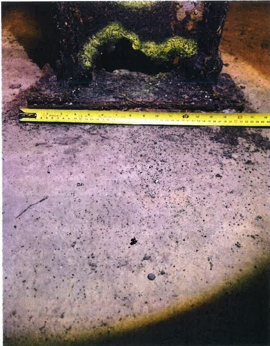
Extensive corrosion at base of support stanchions
