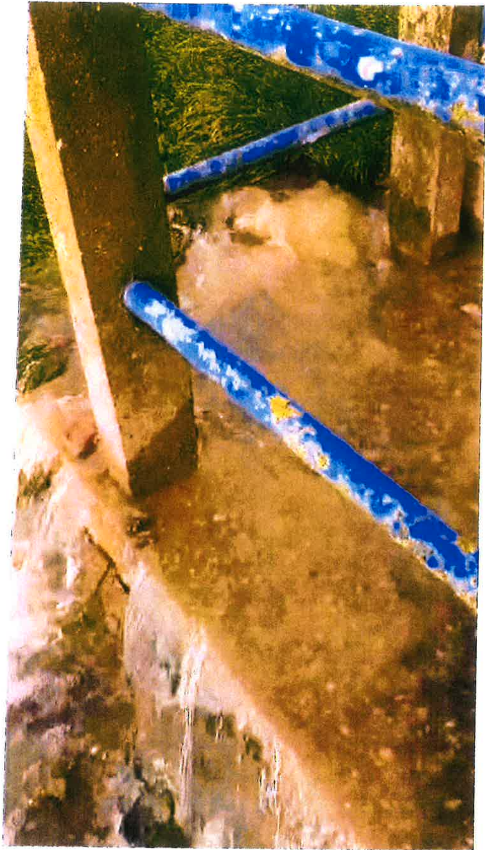
Photo 2 showing where the water was coming through the bank
